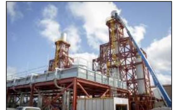
Schofield Barracks, Hawaii: 50 MW Biofuel/Multi-fuel Project operational since May 2018. Full "Islandable" energy capability expected for Schofield Barracks, Camp Kunia and Wheeler Army Airfield
