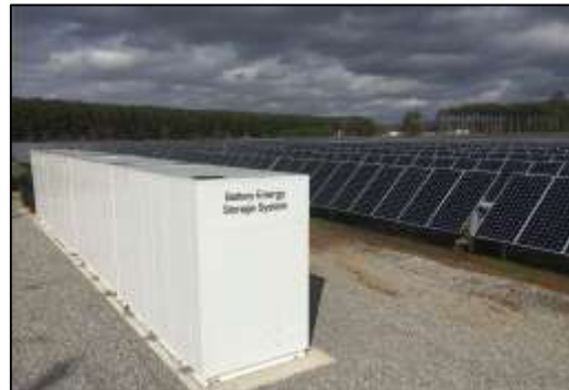
Redstone Arsenal, Alabama: 10 megawatt (MW) alternating current solar project with Army's first privately funded, commercially available battery storage solution
